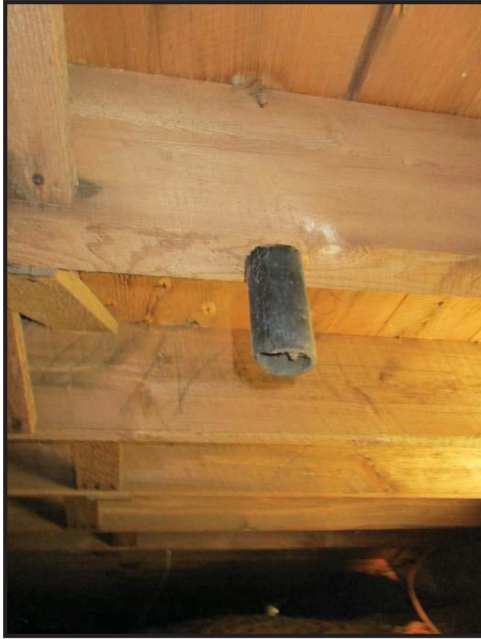
Figure 8 - Floor joist near southeast corner of the building, strength compromised by pipe penetration.
