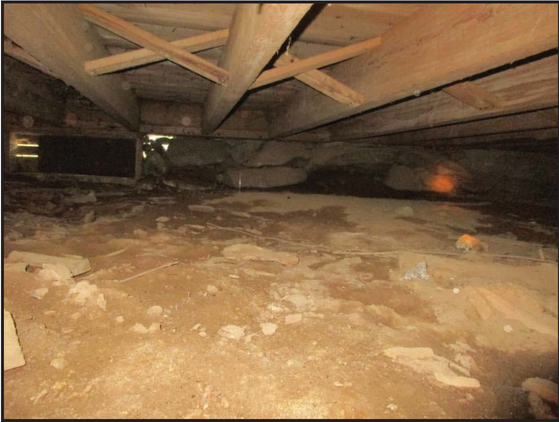
Figure 5 - View of first floor framing. Dirt floor with no vapor barrier was observed within the crawl space. Wood framing appeared to be in fair condition, with little to no rot/moisture damage observed.
