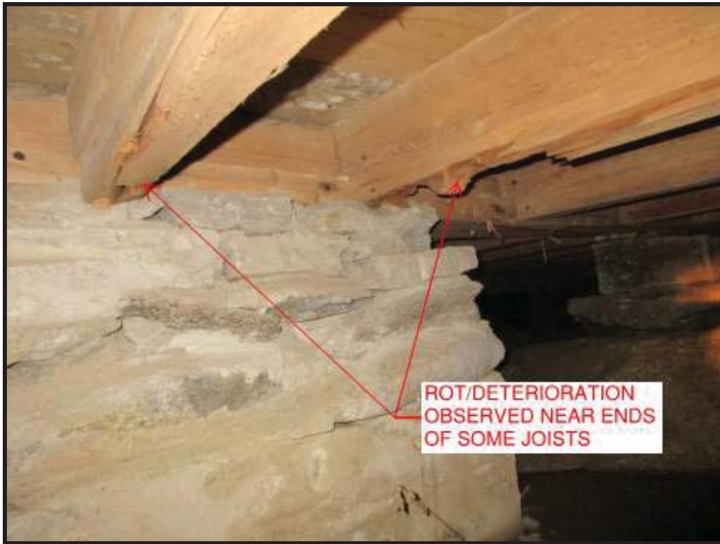
Figure 9 - Damage at ends of joists was observed in a few locations.
